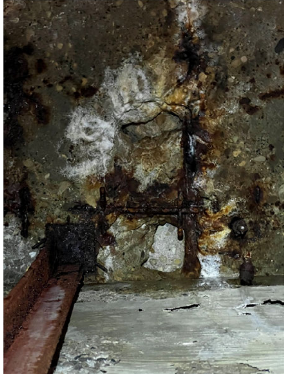
Figure 2: Hanger Attachment and Slab Spall
