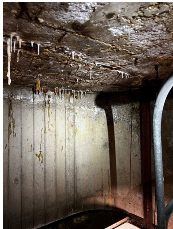
Figure 1: Slab Cracking and Efflorescence
